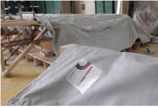
Since last year, the entire daily production of balconies has been treated with Combitherm's thermal concrete mats
